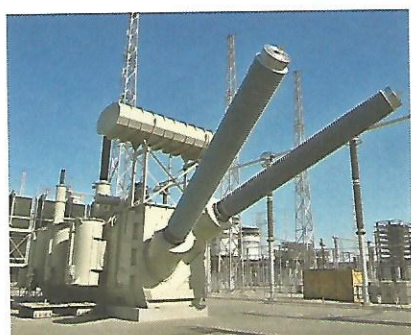
±800kV Oil-SF 6 DC Bushings Hami-Zhengzhou DC Hami Substation Project
