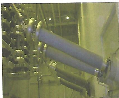
±400kV Oil-SF 6 DC Bushings Jinsu Project, Yulong Converter Station Project
